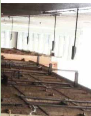
Fig. 7.3134 Wall Mounted Lighting
